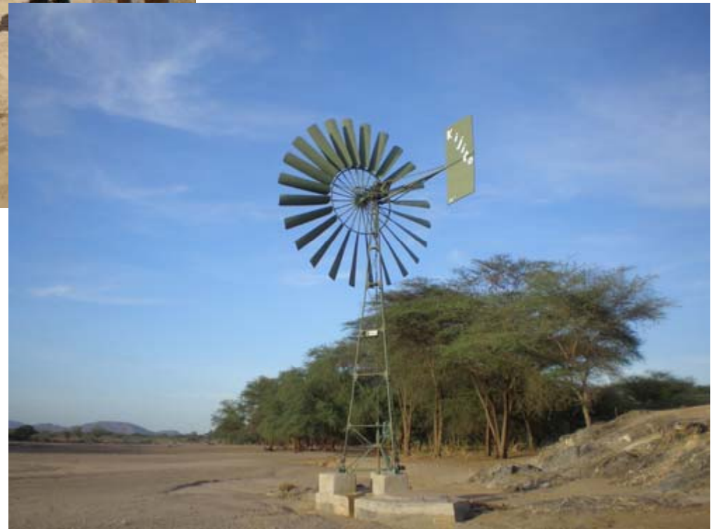
Alternative energy harnessed to pump water from a borehole in Turkana
